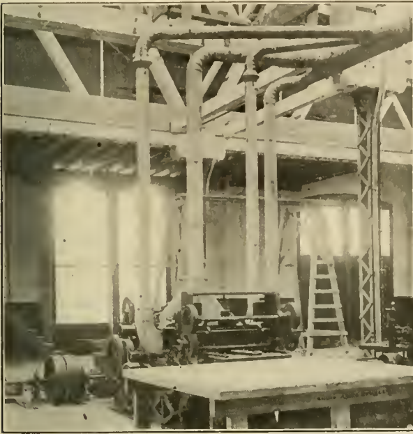
REFUSE COLLECTING PIPES IN WOODWORKING SHOP, CANADIAN PACIFIC RAILWAY, MONTREAL.
